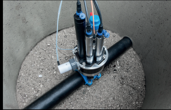
Example of an installation in a manhole
